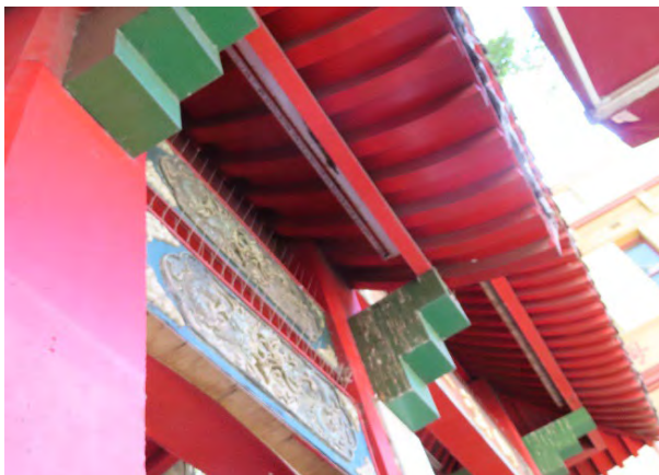
Figure 4.47 Delaminating plywood on the lower decorative panel D.
