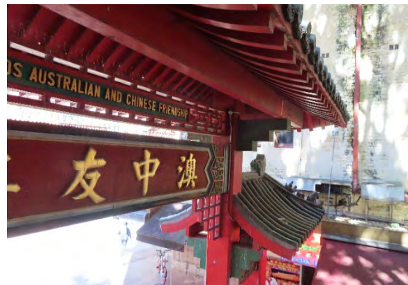
Figure 4.38 Upper decorative panel A with signage sagging (image taken from the north).
