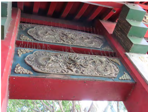
Figure 4.10 Deteriorated plyboard of panels D and E on the eastern bay .
